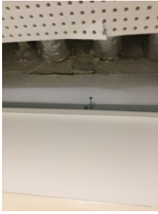
Evidence of shrinking fire stopping.
