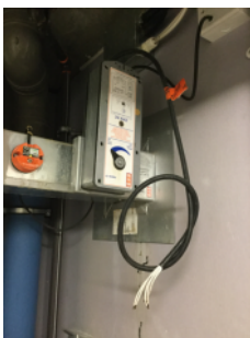
Fire damper in the riser cupboard top floor.
