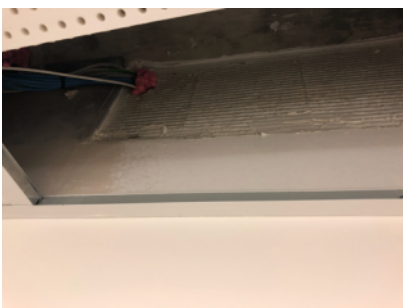
Poor fire stopping
