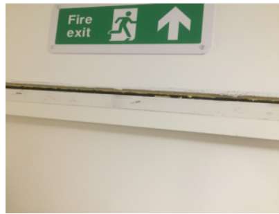
4th floor staircase door frame before fire stopping.
