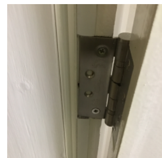
Missing screws on ground floor staircase door
