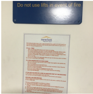
Fire action notice ( rear entrance)
