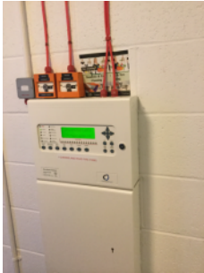
Smoke control panel at the rear entrance of 1 Queensland.
