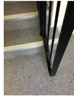
Evidence of smoking, base of stairs, ground floor.
