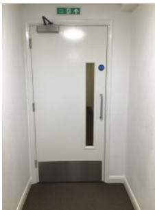
Corridor fire door fitted with intumescent strips only
