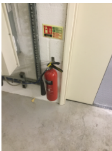
CO2 Extinguisher in ground floor pump room.
