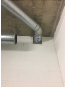
Duct within bin store - cooler air pulled naturally into adjacent pump room
