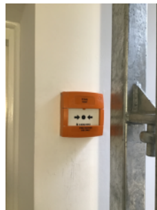
Staircase ventilation override
