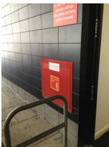
Dry riser inlet
