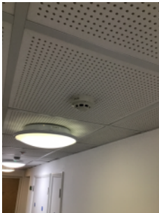
Corridor smoke detector for AOV actuation
