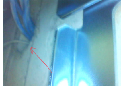
Penetrations into lift shaft without fire stopping, 10th floor.
