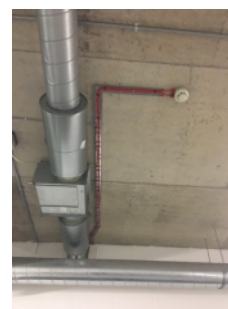
Duct within bin store, with fan pulling warm air out of pump room
