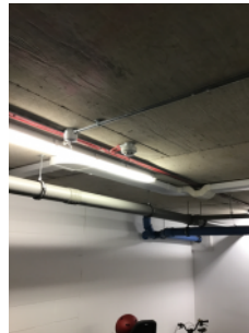
Bike store smoke detector
