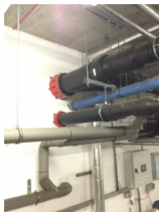
Fire collars in the plant room.
