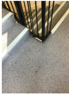
Evidence of smoking, 1st floor landing.
