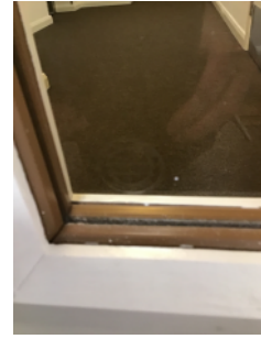
Fire glass UK mark in corridor fire door
