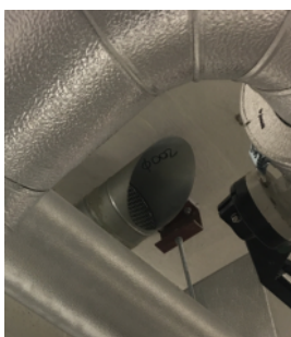
Ducting within pump room ground floor - warm air inlet
