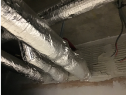
Example of good fire stopping, above ceiling, above entrance to flat 25
