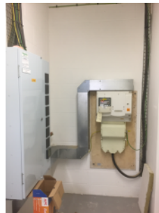
Electrical cupboard 2 ground floor
