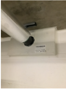
Fire stopping in bike store
