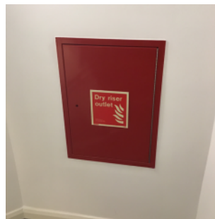
Example dry riser outlet.
