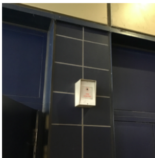
Rear exit door override.
