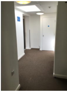
Normal lighting levels on 10th floor
