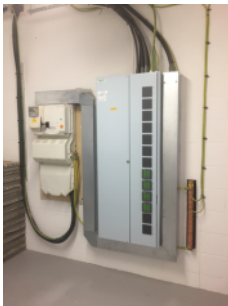
Electrical cupboard 1 on ground floor
