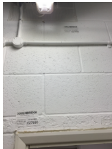
Evidence of recent fire stopping being carried.
