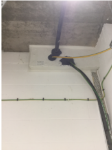
Version 8 - 1/4/20 Evidence of fire stopping
