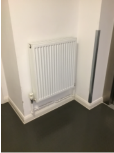
Hot water radiator in lift lobby on 1st floor
