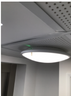
Emergency lighting unit in corridor
