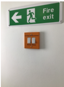
Corridor smoke extraction controls, coated in stairwell
