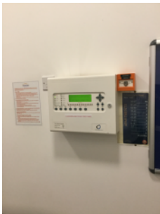
Smoke control panel in the rear lobby.
