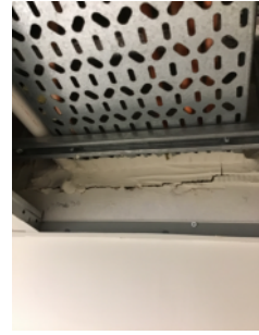
Example of shrinking, cracked fire stopping - 3rd floor riser.
