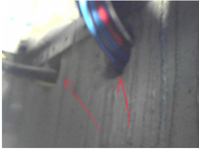
Penetrations into lift shaft without fire stopping, 10th floor.
