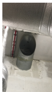
Ducting within pump room ground floor - cool air inlet
