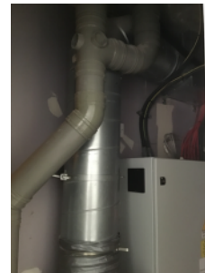
Ducting from bin store, seen in riser cupboard 5th floor.
