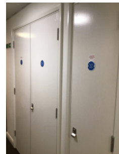
Riser cupboards in corridor
