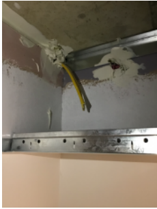
Example of poorly applied fire stopping, above staircase door, 3rd floor.
