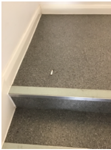
Evidence of smoking, 1st floor.
