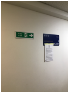
Fire exit signage
