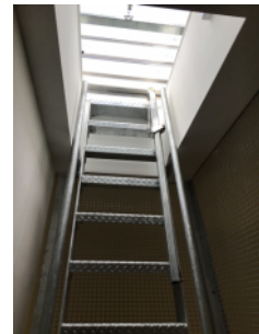
Staircase AOV at head of stairs
